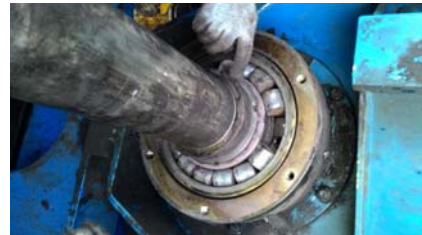
Gbr. 8 Bearing Rusak
