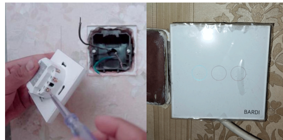
Gbr 2. Instalasi Smart Wall Switch
