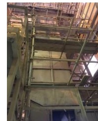
Gambar 2. Bucket Elevator M2202 (Sumber : PT. XXX)
