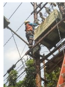
Figure 4. Transformer Connection Inspection
