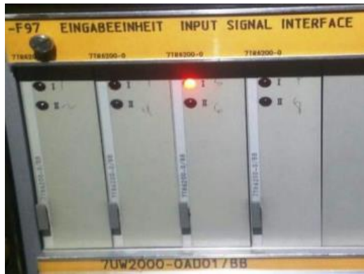
Figure 4. GTG No.3 HV Line protection trip alarm
