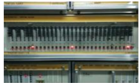
Figure 5. STG No.3 HV Line protection trip alarm
