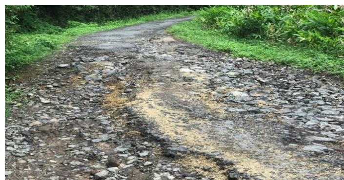
Figure 1. The damage at the Kopeng 1 incline (2024). Resource: Author, 2024
